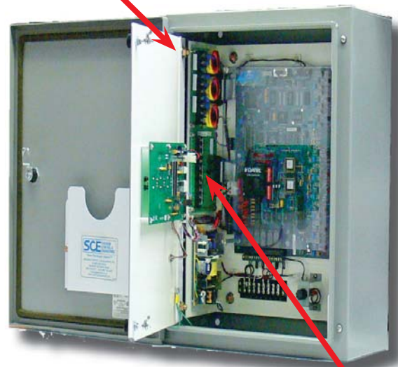
6PTP2 Potential Transformer Interface
