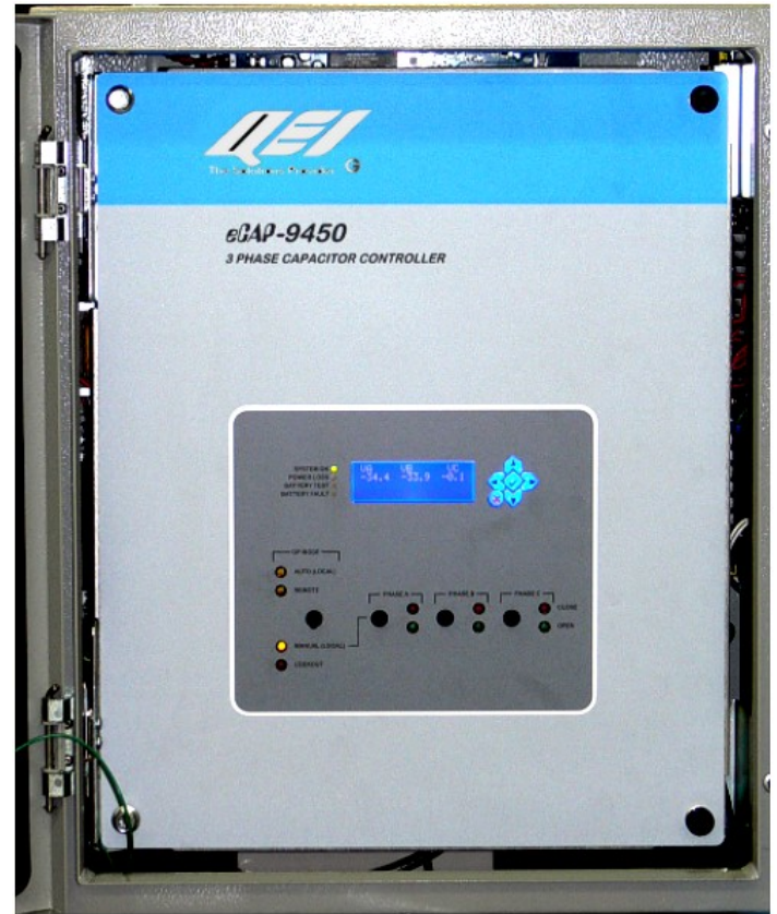
Front Panel LED Readout Permits Quick Review of Controller Operation Without the Need for a Laptop
