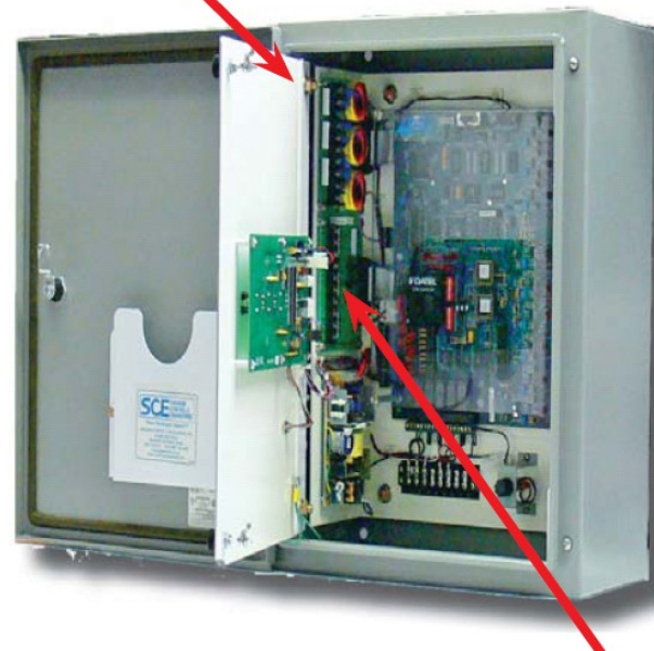
6CTP2 Potential Transformer Interface
